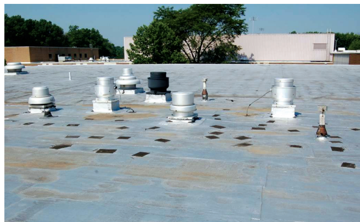
Portion of OFHS Roof BEFORE Phase 1 Repairs
